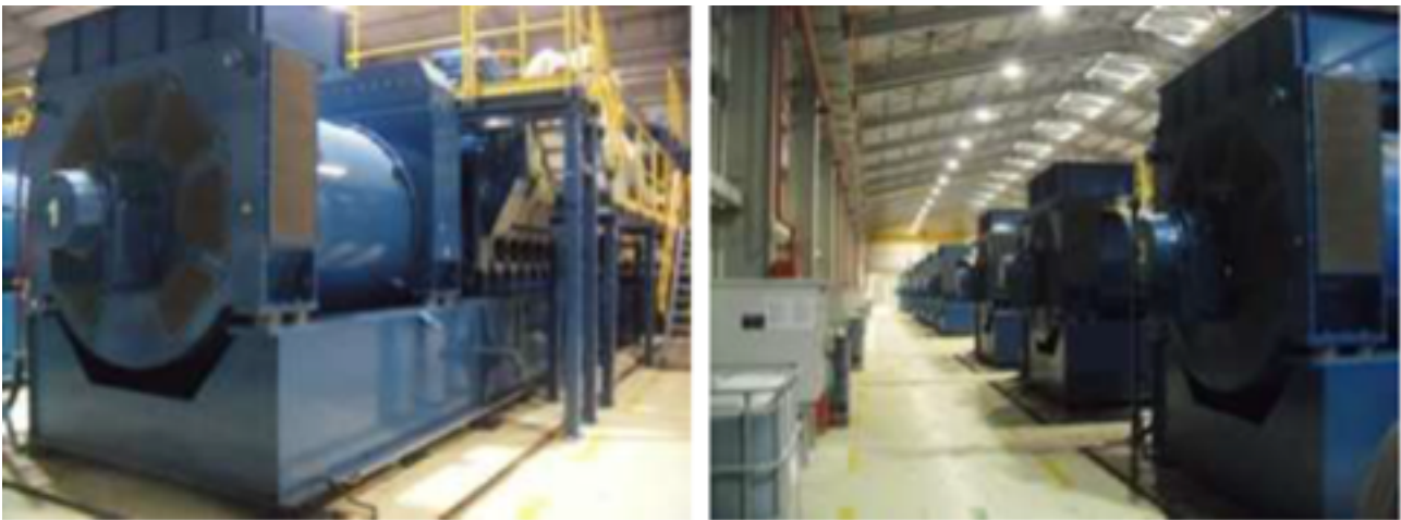
Gas Engines, Alternators, incl. its Equipment
