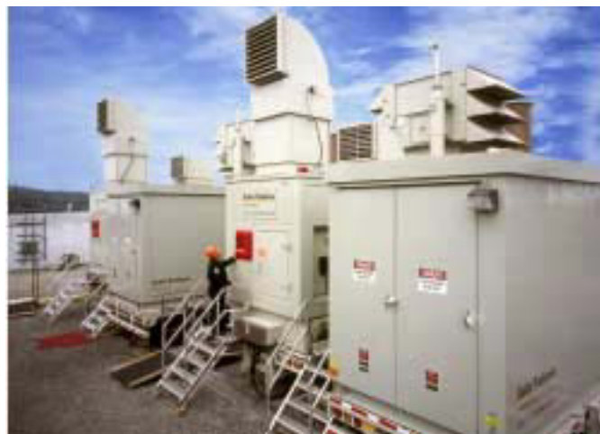
Sited Configuration of Taurus 60 Mobile Power Unit
